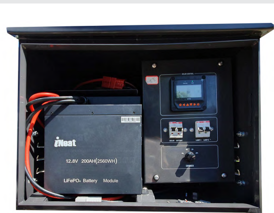
Battery and Control Box
