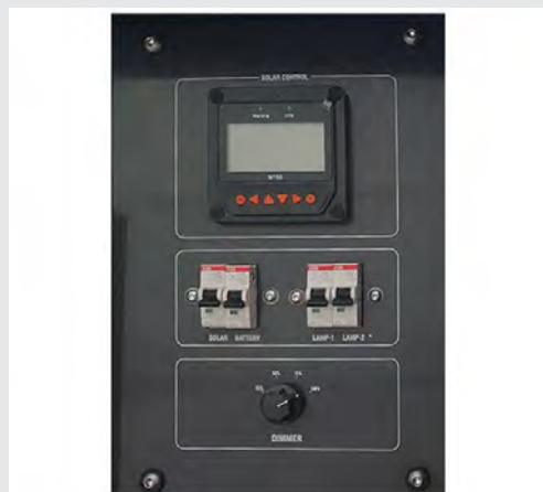
System Control Panel
